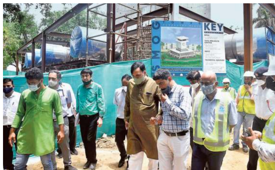
Delhi Environment Minister Gopal Rai at the construction site of a smog tower at Connaught Palace in the city on Thursday. *SHIV KUMAR PUSHPAKAR
