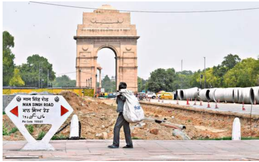
Construction work of the Central Vista project in full swing in New Delhi. ■SHIV KUMAR PUSHPAKAR
