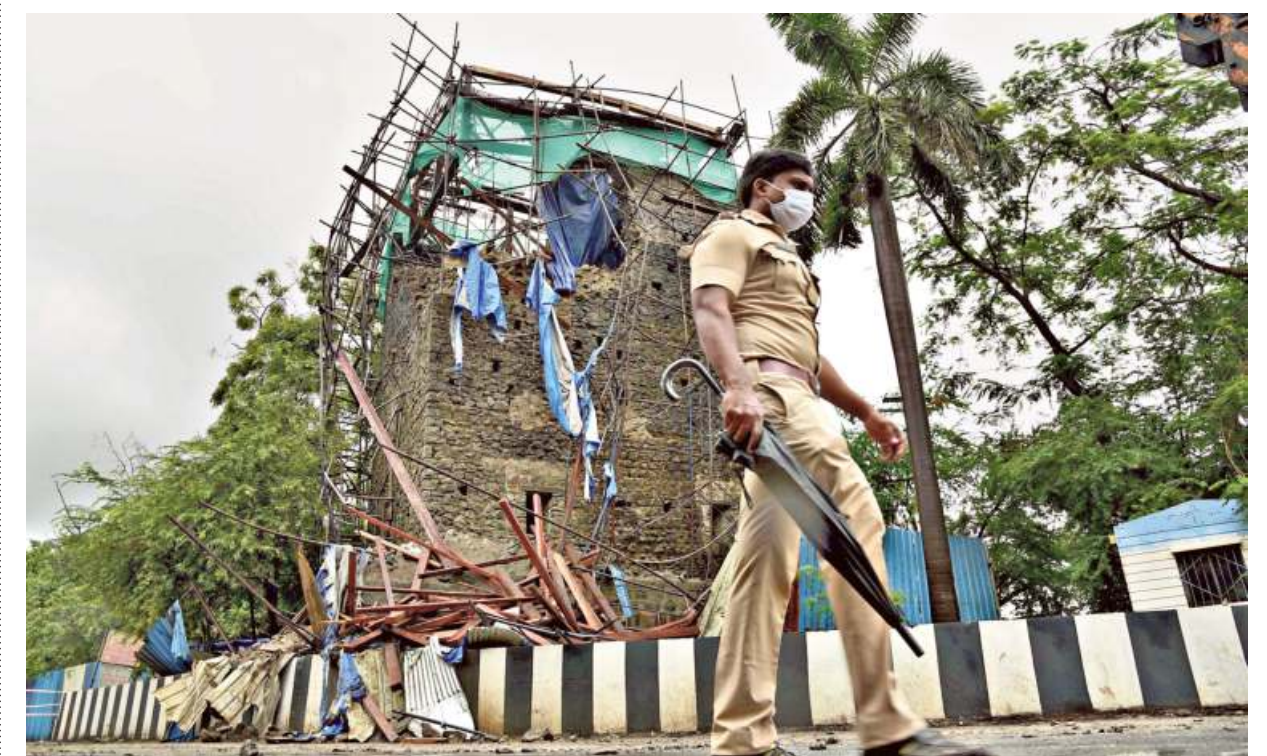
Blown away: The remains of a steel scaffolding erected for the restoration of Belapur Fort after it collapsed due to heavy rain in Navi Mumbai on Saturday. A passenger travelling in an NMMT bus sustained injuries in the incident. ■ PTI
