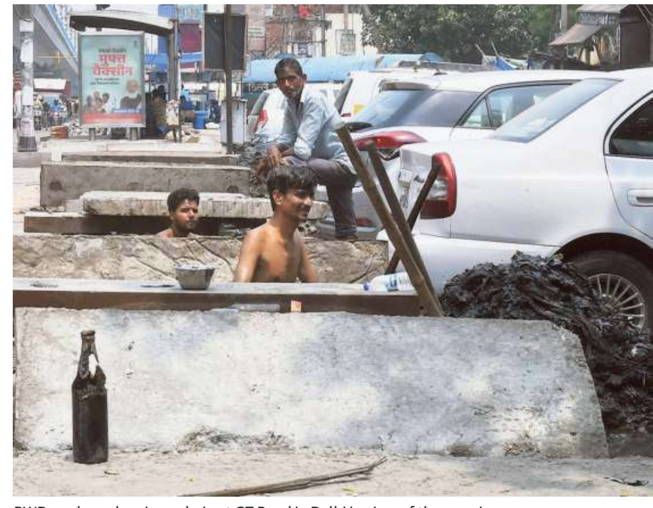
PWD workers cleaning a drain at GT Road in Delhi in view of the ongoing monsoon season. •SUSHIL KUMAR VERMA
