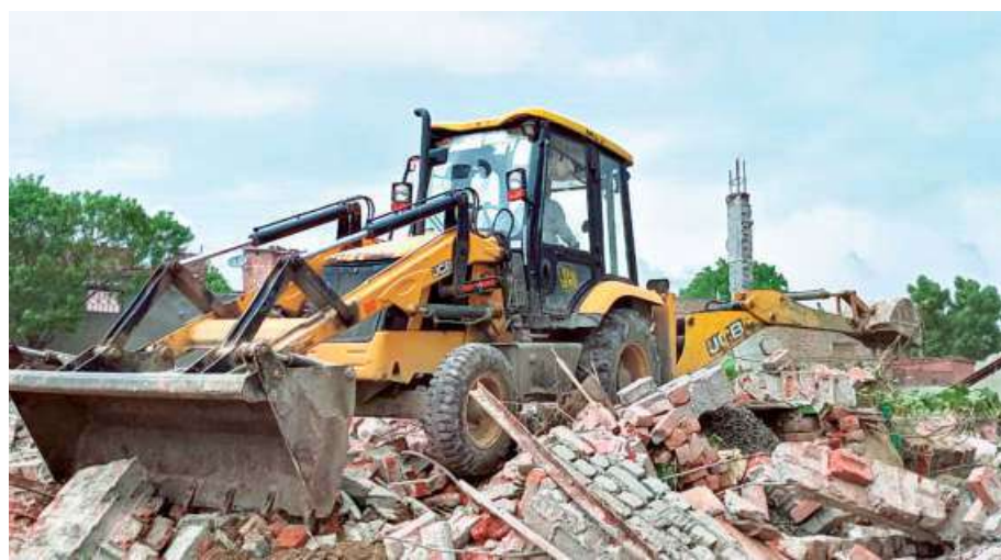
Municipal Corporation of Faridabad kicked off demolition on Wednesday. The drive was, however, called off midway due to heavy rain. *SPECIAL ARRANGEMENT
