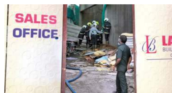
Tragedy: Rescue workers at the under-construction building in Worli, where a lift collapsed on Saturday. ■EMMANUEL YOGINI
