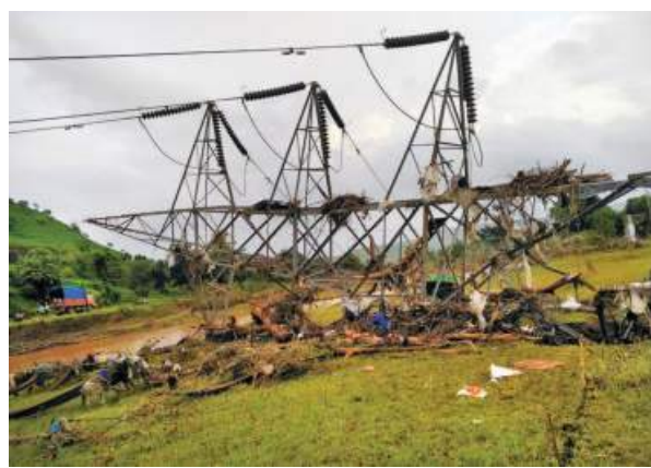
Knocked down: Two high-voltage towers of MSETCL collapsed following heavy rainfall on Thursday. ■SPECIAL ARRANGEMENT
