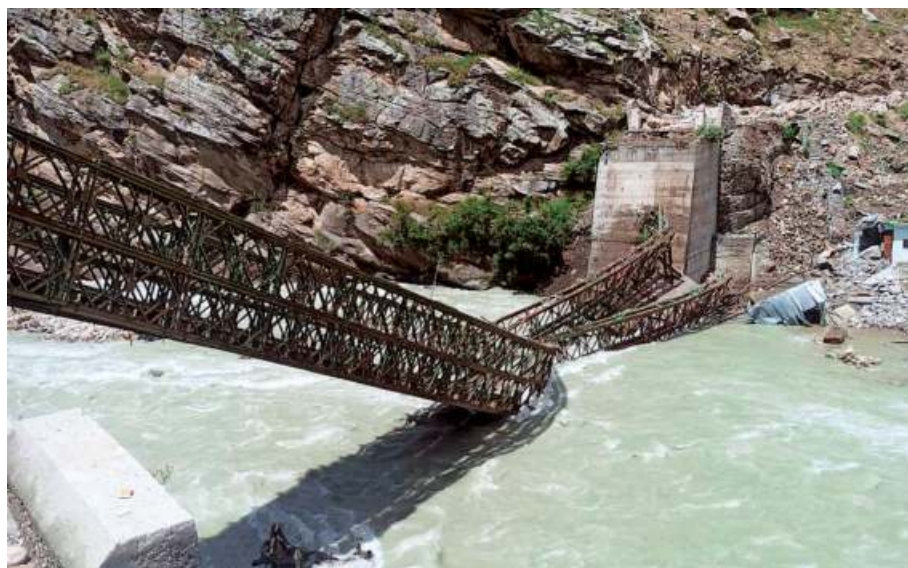
Disaster site: The collapsed bridge seen after multiple boulders hit it during a landslip at Basteri in Kinnaur district of Himachal Pradesh on Sunday. •PTI
