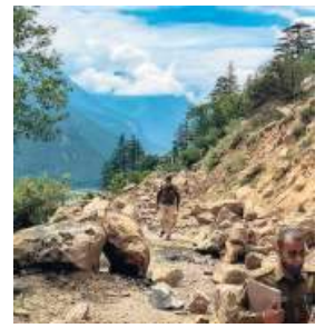
A stretch of road that was damaged by the recent landslide in Kinnaur.
