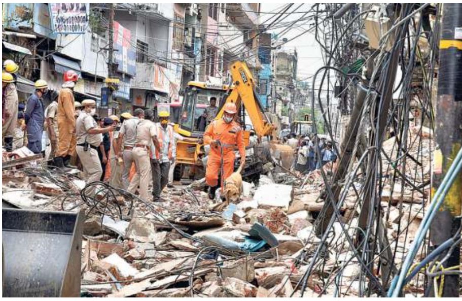
Rescue work in progress at a building collapse site in north Delhi's Sabzi Mandi on Monday.
