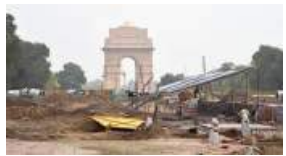
The work is expected to be completed ahead of the R-Day parade next year.
