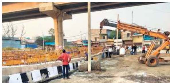
A crane being used to remove the barricades placed near the farmers' protest site at Tikri border. ■ SPECIAL ARRANGEMENT
