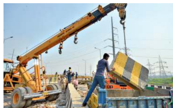
Free passage: Barricades put up by the police on the Delhi-Meerut Expressway being removed on Friday. ■ R.V. MOORTHY
