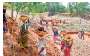
A file photo of workers engaged in desilting work in Visakhapatnam. • K.R. DEEPAK
