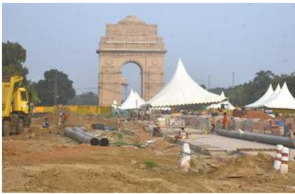
Mega project: Construction work at Rajpath as part of the Central Vista Avenue redevelopment. • FILE PHOTO
