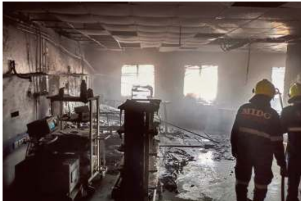
Fire fury: The fire-ravaged ICU of the district civil hospital in Ahmednagar of Maharashtra on Saturday. • AFP
