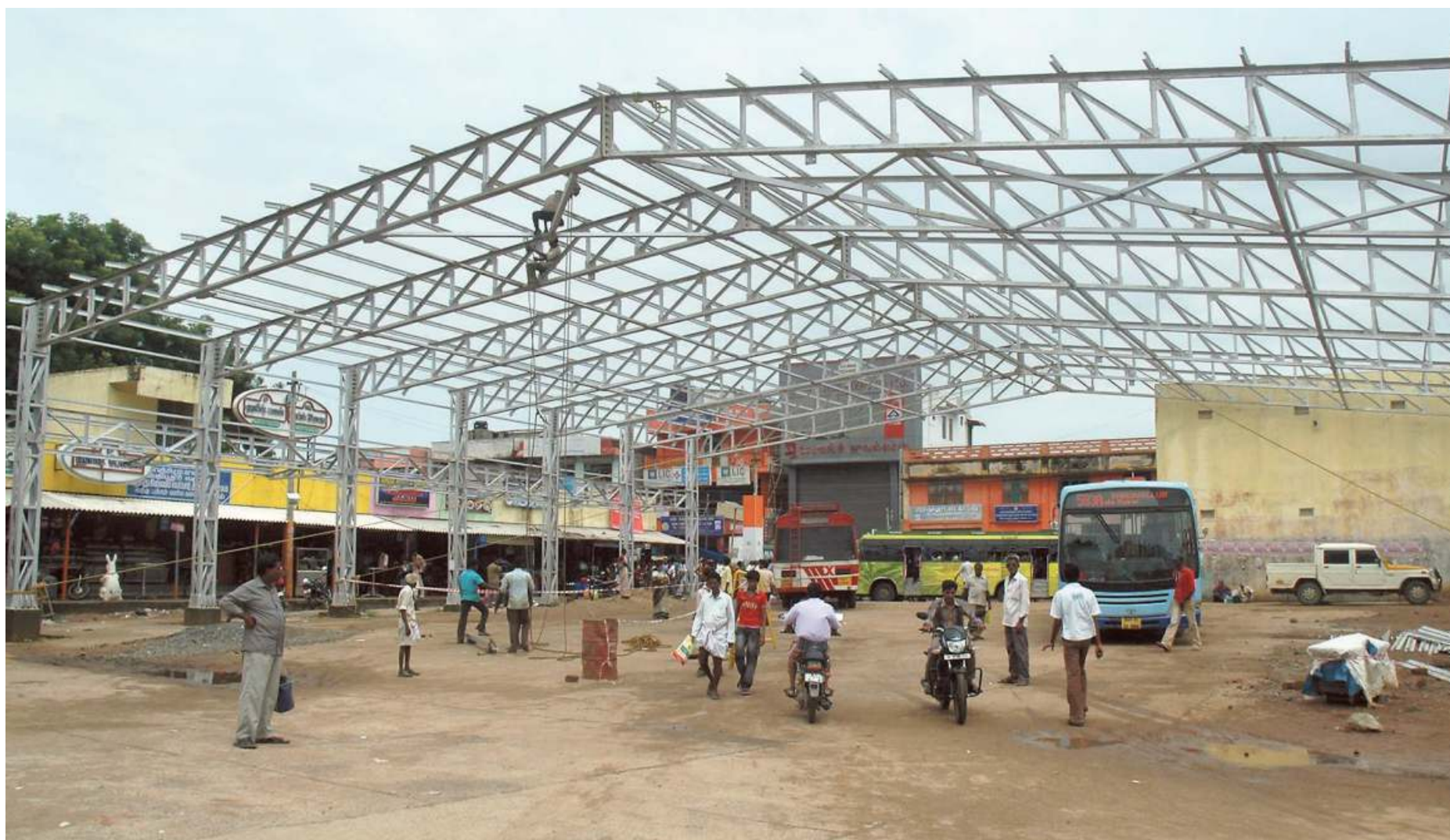
Work in progress: A bus shelter under construction under the MP Local Area Development scheme at Sriperumbudur in Kancheepuram district, Tamil Nadu, back in 2011. • JOTHI RAMALINGAM B.
